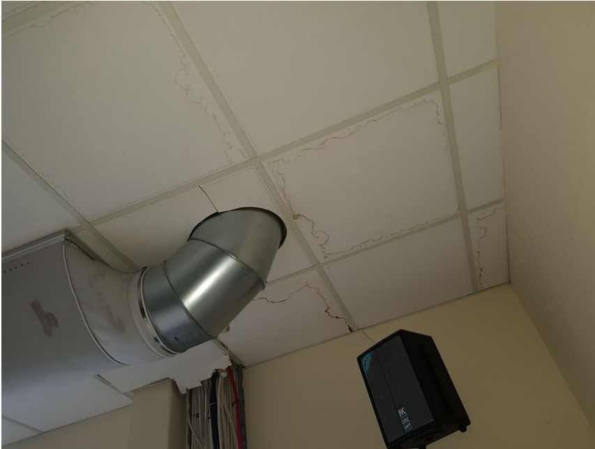
Gym, plan 1 – Fuktskador i innertaket runt tilluftsdon
